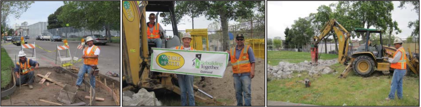
Crew (left to right) Ramon Figueroa, Victoriano Martinez, Jorge Gomez, Dave Burgeno and Milton Vasquez prepare site for the installation of playground equipment
